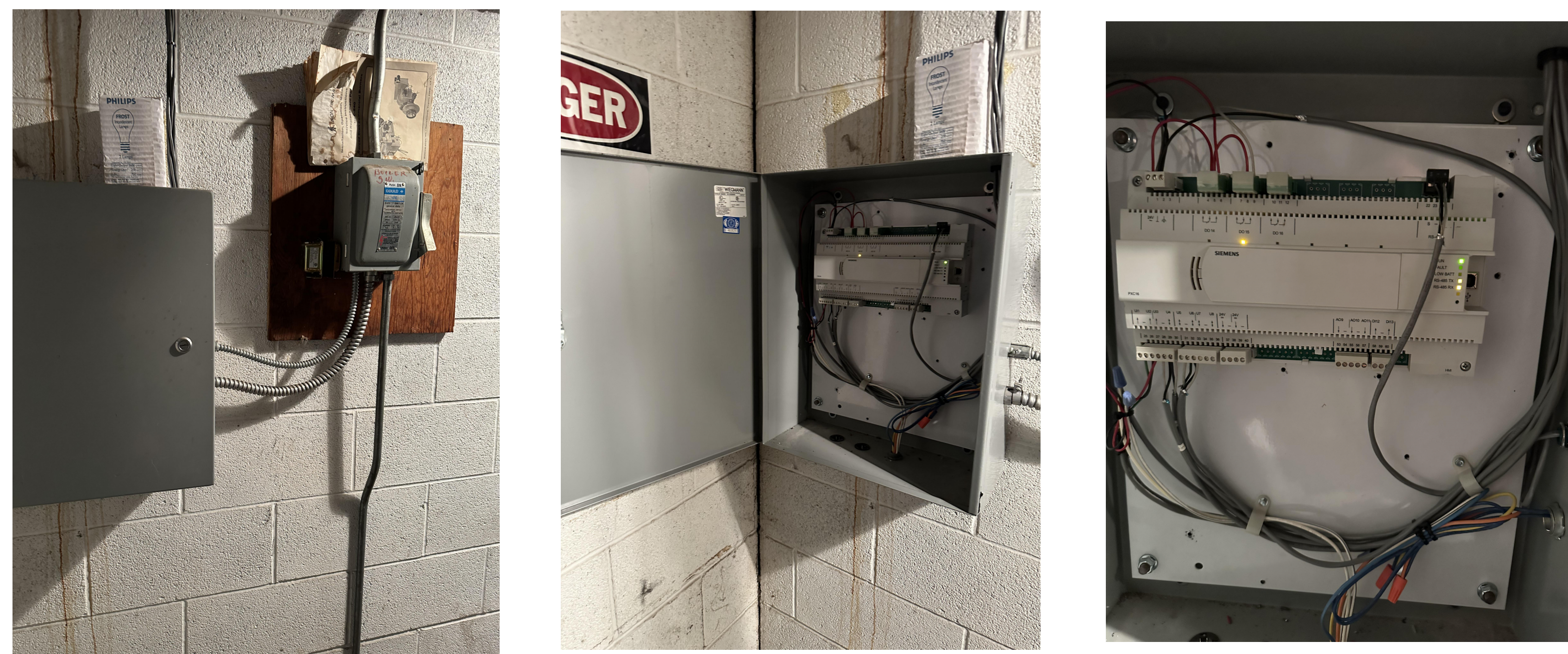
CONTROL PANEL PICTURES
